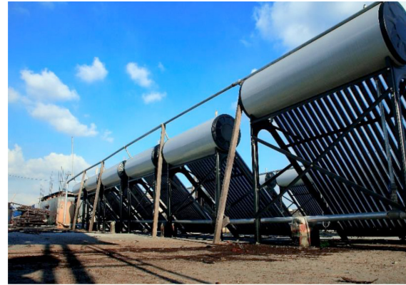
Figure 6: Solar collectors installed in a tannery under UNIDO project in Bangladesh. Source: UNIDO
