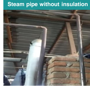
Steam pipe without insulation
