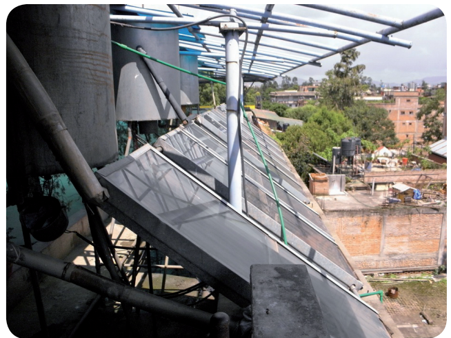
Solar water heaters implemented by SEID
