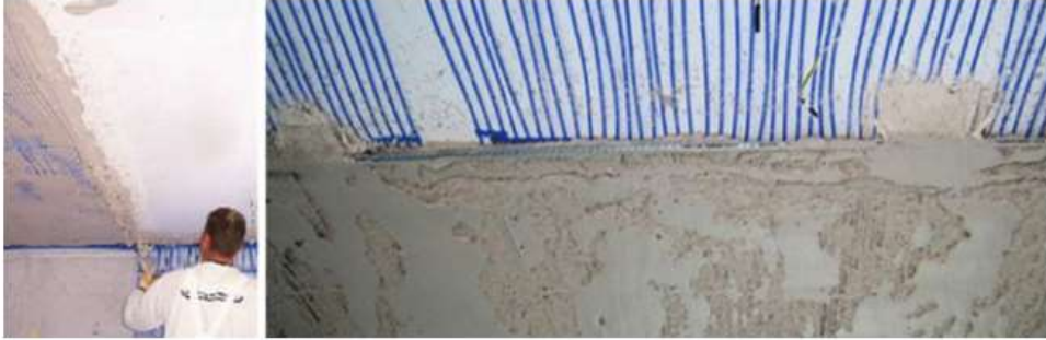
Figure 31: Installation of the active-chilled ceiling system containing PCM-enhanced plaster and plastic micro-tubing - Fraunhofer ISE, Germany. (Kośny, 2015, p.43)
