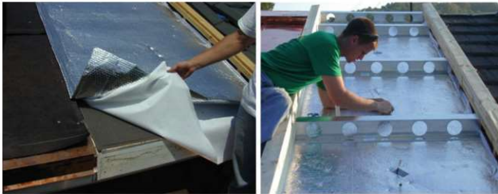
Figure 32: Fig. 18: Construction details of a roof assembly containing, reflective insulation, and subventing air channels, followed with two PCM insulation systems produced by Outlast, USA. (Kośny, 2015, p.46)
