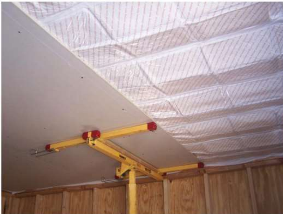
Figure 35: Installed BioPCM Mat in the Ceiling. ( Muruganantham, 2010, p.16)
