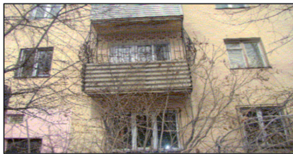
A. Balcony of an apartment building was covered by asbestos panel
